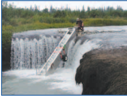
The completed steppass provides a channel for coho salmon to swim up and over the impassable falls.
