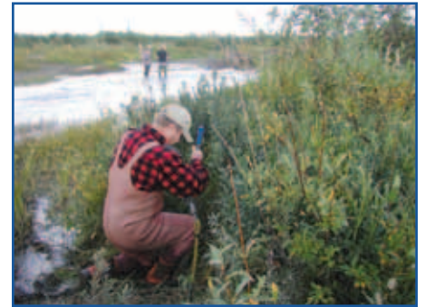
Project Technician, Ron Carlson, tightens the cables that help support the steeppass.
