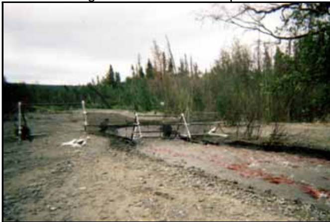
The weir at Bear Creek on Tustumena Lake is now surrounded by a barren landscape, due to the severe flooding during the fall of 2002.
